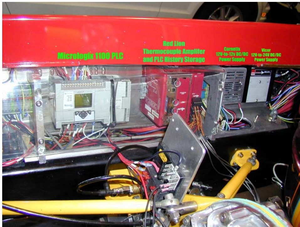
Location of PLC, Red Lion Data Station and DC/DC Power Supplies
